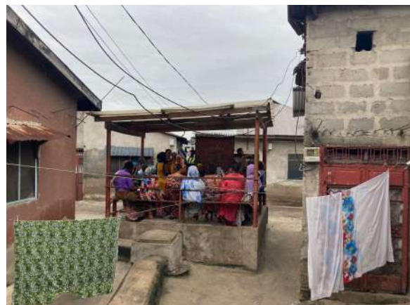
One of the biogas chambers that are part of the simple sewage and biogas generation system. Vigunguti, Dar es Salaam. Photo: Priscila Izar, 19 April, 2024.
