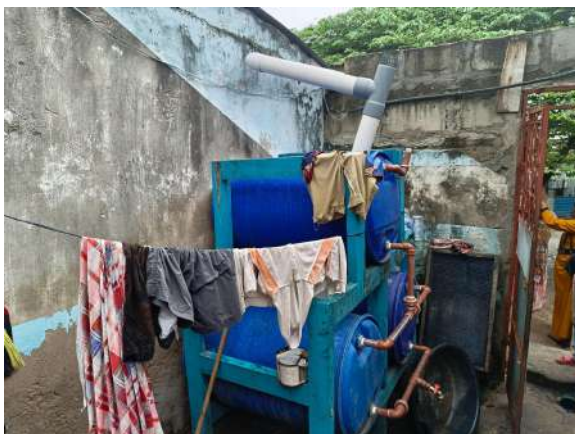
Rain catching system developed by CCI and PANAKUNA. Vigunguti, Dar es Salaam. Photo: Paula Santoro, 19 April, 2024.
