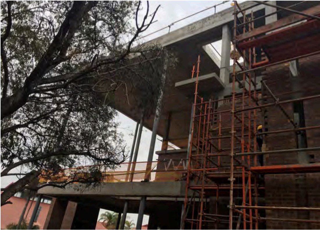
Fig. 13.19: University of Mpumalanga Campus Building L005 – ICT Academic Building. View of construction June 2017.
