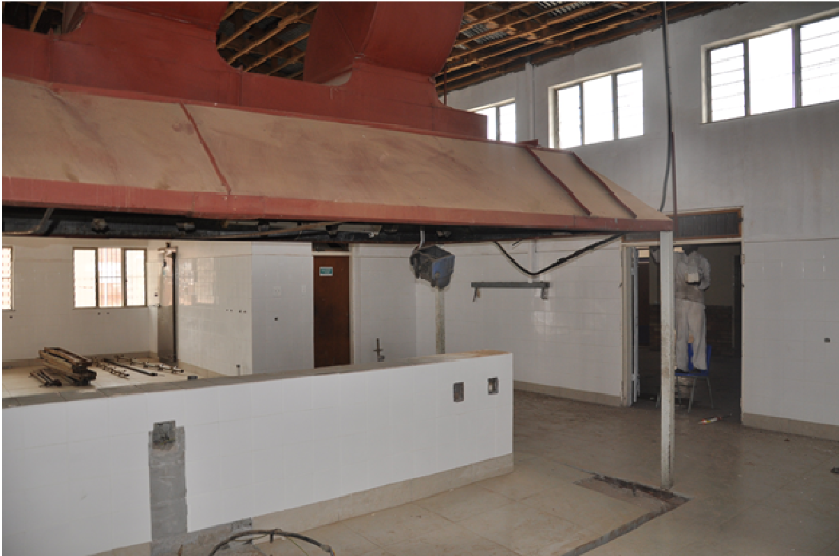
Fig 6.29: University of Mpumalanga Siyabuswa Campus renovation and upgrade of the existing dining amenities.
